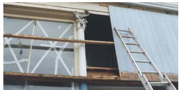
By removing these panels from a building in Sharon, WI, the original transom windows were exposed once again for very little cost.
