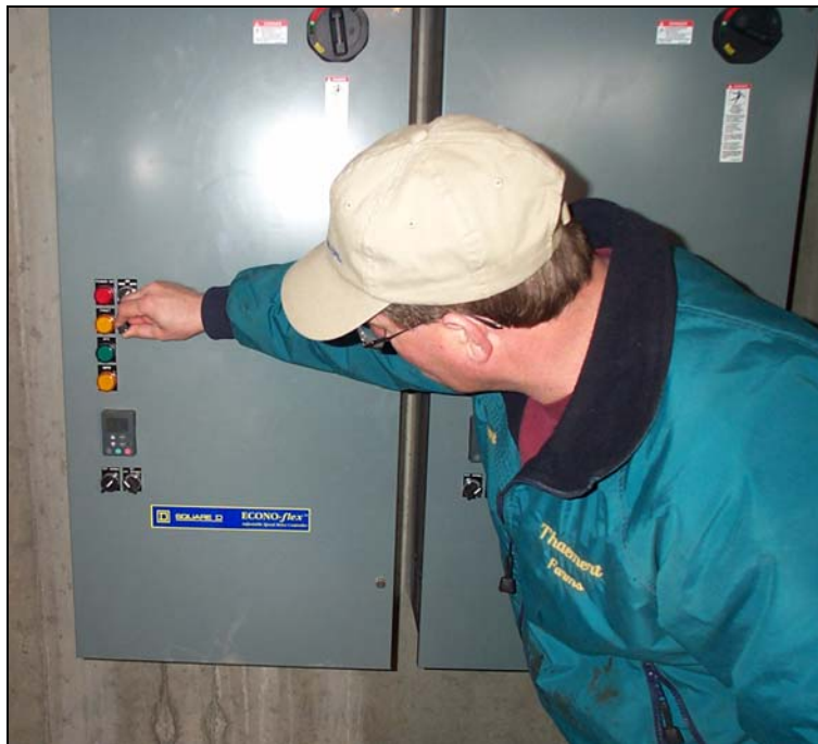
Figure 8: VFDs with Bypass Contactors, Thaumert Farms
