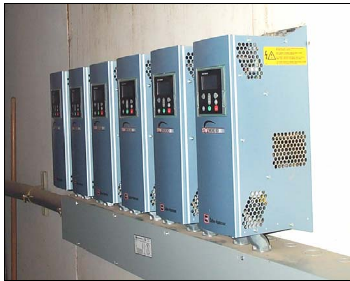
Figure 5: VFDs at Lamb Weston 1, Warden WA
