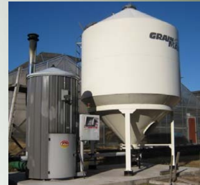
Pellet boiler & bin
