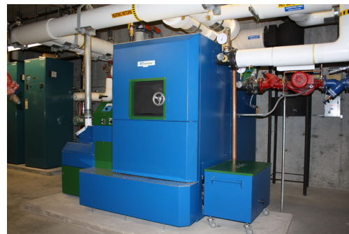
Advanced Climate Technologies built the first made-in-NYS commercial high-efficiency wood pellet boiler, which was installed at The Wild Center. Photo courtesy of The Wild Center
