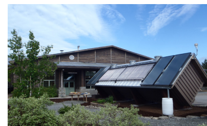
The pellet storage bin at The Wild Center is a re-purposed shipping container that also supports a solar thermal hot water system. Photo courtesy of NYSERDA
