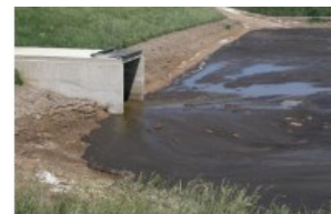
Non-enclosed manure storage should be assessed to determine employee exposure to safety and health hazards.
