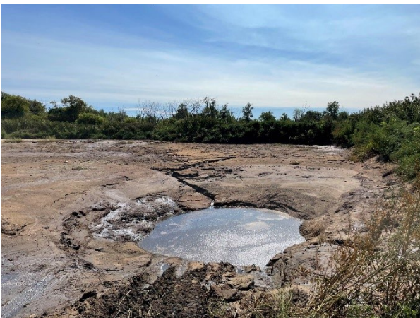
Photo 20: What the overflowing/leaking manure storage structure looked like in September 2022 with most of the liquid pumped out. NOD grant funding was used to properly close this facility.
