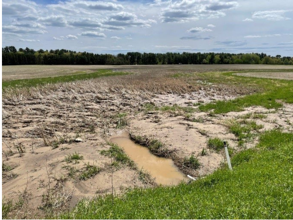
Photo 41: Sediment deposited in wetland on other side of road
