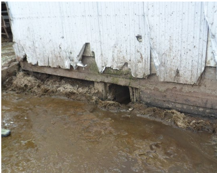
Photo 42: Underground pipe inlet draining barnyard runoff
