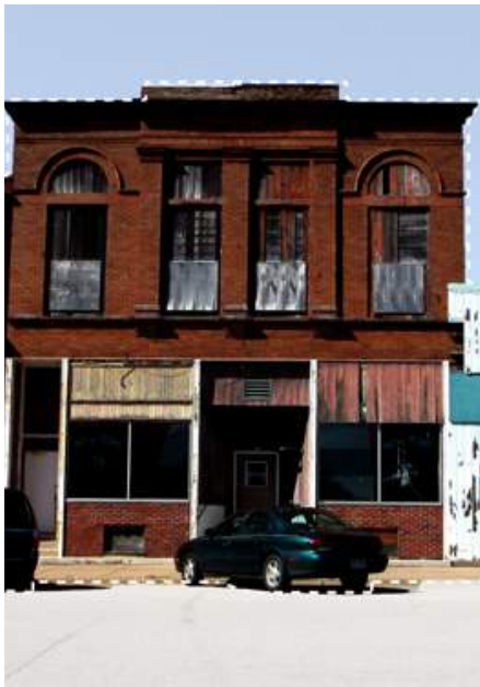
Existing Characteristics: Degrading Facade
