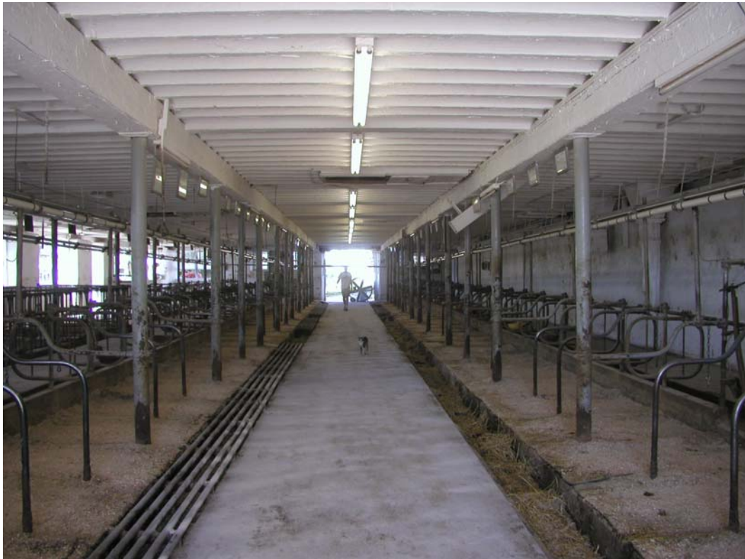
Figure 2. Interior Photo of Two Story Dairy barn with two rows of posts and beams.
