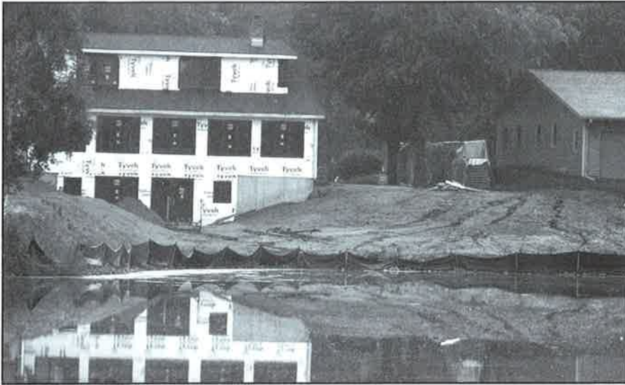
The intent of mitigation is to offset the impacts to water quality, near-shore aquatic habitat, upland habitat and natural scenic beauty from proposed construction projects within the shoreland zone.
